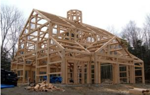
Figure 1-27. Timber-frame building designed by Steven Knox and built by Connolly & Company, Edgecomb, Maine. Image from http://stknox.com/images/StudioBarnFrame.JPG .
