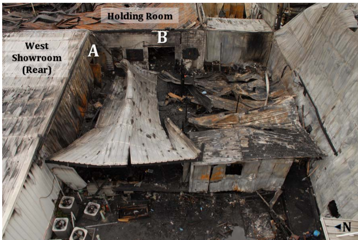
Photo 2: Post-fire view of the loading dock. Note the double doors (A) connecting the loading dock to the west showroom at the upper left and the open garage door (B) in the concrete block wall between loading dock and the holding room. (Photo courtesy Bill Murton, Charleston Police Department)
